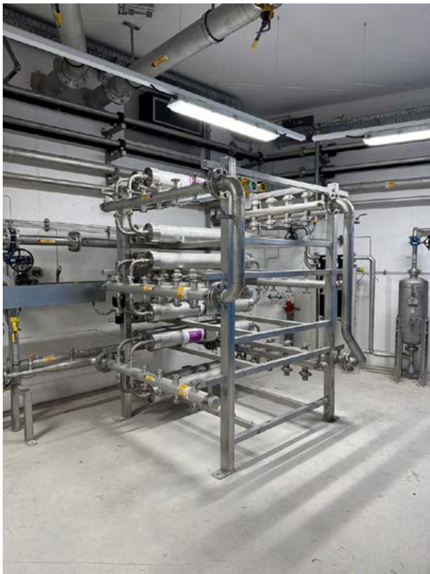
Membrane plant of the new naturemade star-certified biogas plant in Basel (photo: ProRhenon)
